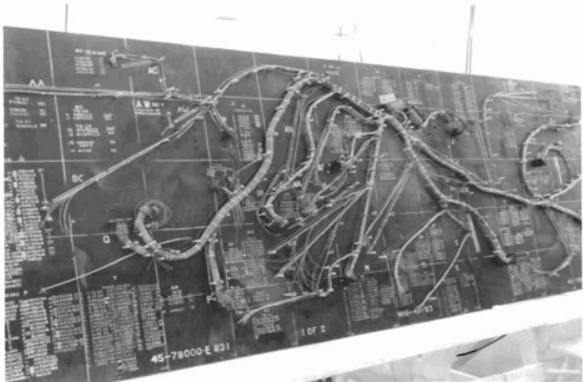
Figure 3 Electrical motherboard for wiring assembly. Source: Box 75, Project Mercury Photographs, Entry No. 70, History Office Source Files, RG 255, NARA-Southwest. (NASA)
